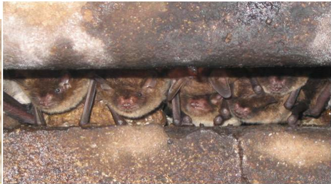
Photo 2: Visible bats within an expansion joint
